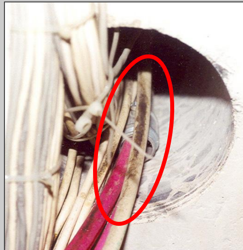
Staining from mice on electrical wiring
