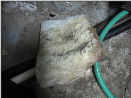
Evidence of mice in the attic insulation and floorboards
